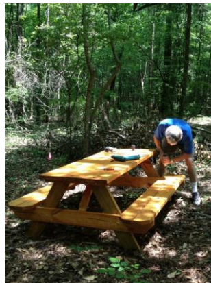
2. The picnic area (2 tables) on a fossilized concrete slab, faces the play fort, next photo. More tables and benches are in the works for this and other areas.
