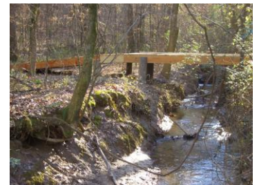
4. Now nearing completion, the foot bridge located about ¾ of the way to Yellowleaf Creek. Work remains on railings and north side ramp. More bridge work pics are on the website.
